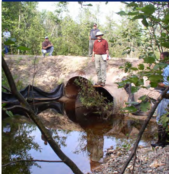
Huron Pines staff and volunteers study the effects of a road/stream crossing on a stream.
